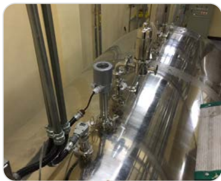
Water purification barrel
