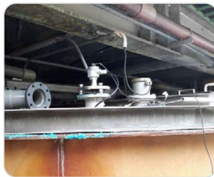
Copper sulfate storage tank
