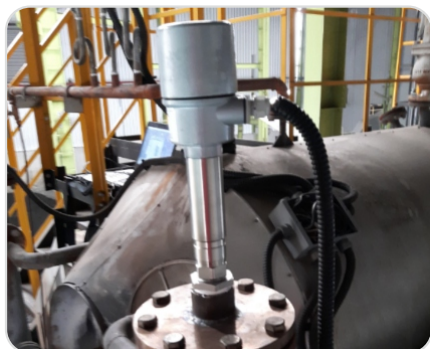
High temperature boiler
